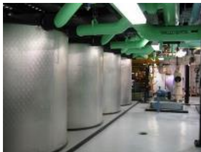
Thermal energy storage battery “Storage Source Heat Pump”
